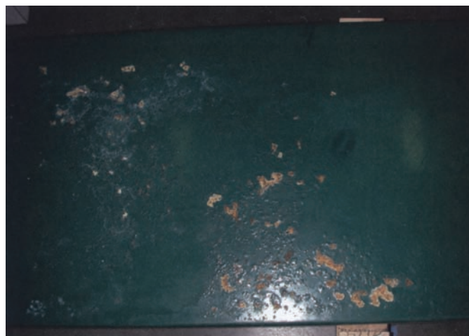
FIGURE 7B Detail of figure 7A showing corrosion.
