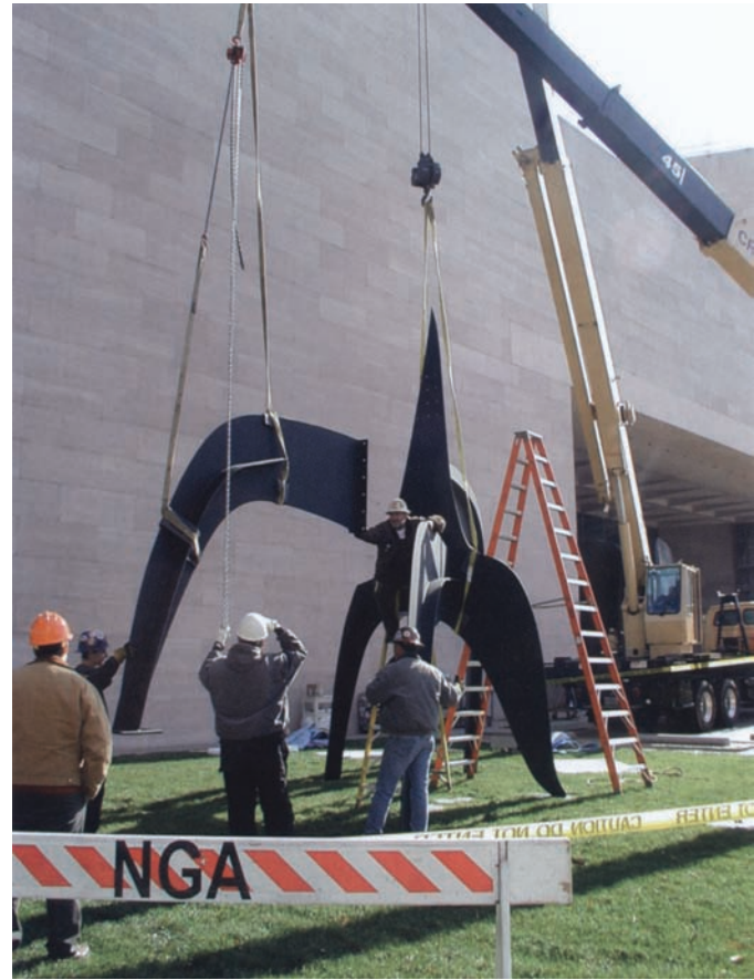
FIGURE 3 Installation in November 2004 of Tom's by Alexander Calder. The adapted paint's superior resistance to weathering should make this type of major disruption and expense far less frequent. Photo: Abigail Mack. © Calder Foundation.
