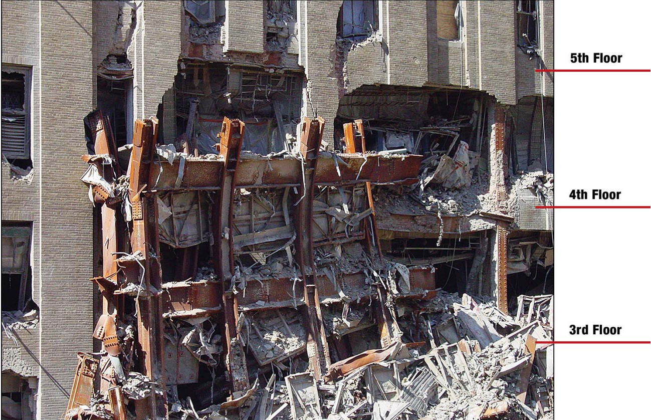
Figure 7-7 Verizon building – damage to east elevation (Washington Street) due to WTC 7 framing leaning against the building.
