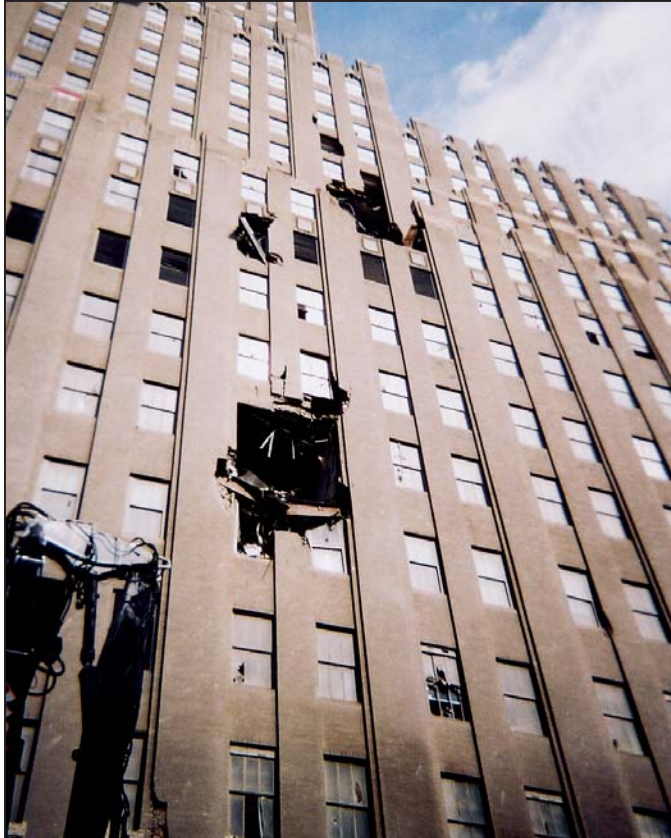
Figure 7-10 Verizon building – damage to south elevation (Vesey Street).
