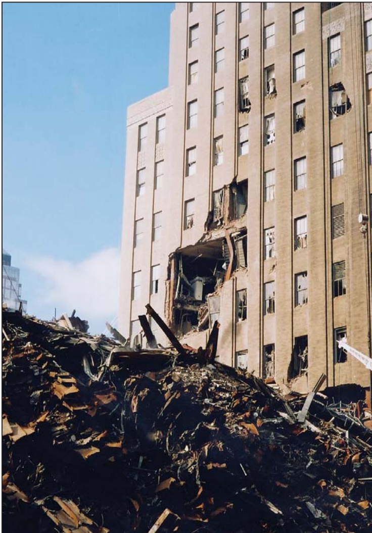
Figure 7-6 Verizon building – damage to east elevation (Washington Street).
