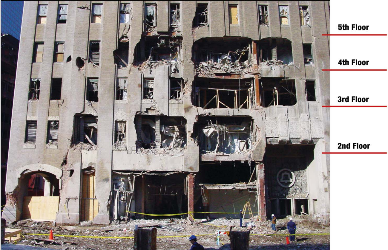
Figure 7-8 Verizon building – damage to east elevation (Washington Street).
