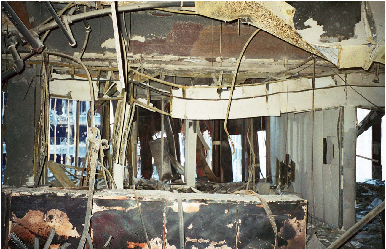
Figure 7-5 Interior damage at floor 20 of WFC 3.
