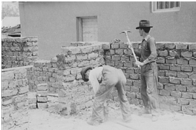
Constructing an adobe building, Penasco, New Mexico. Workers using an informal labor plan.
