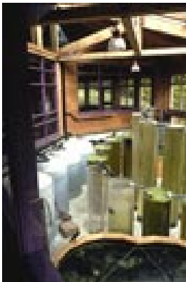
Biological Sewage Treatment
