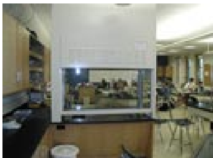
Demonstration Fume Hood
