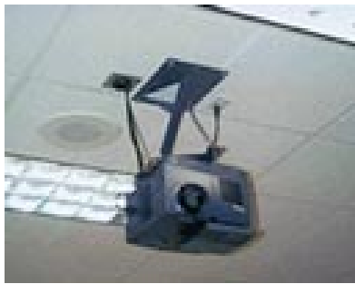
Ceiling Mounted Projector
