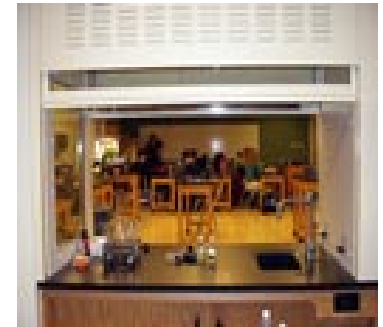
Fume Hood Between Lab and Prep Room
