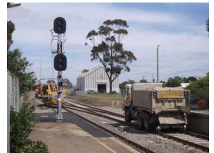
A hi-rail tipper prepares the top ballast beside one of the new signal masts
