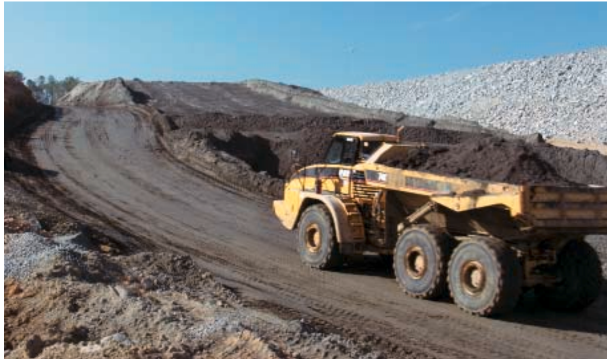
A truck hauls ash that will be used to produce roller-compacted concrete.
