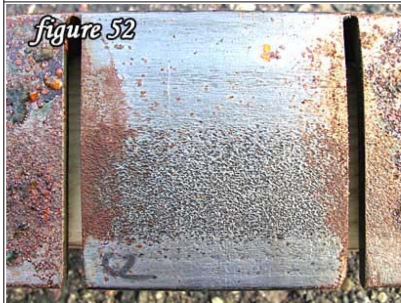
Serious rust has formed where the salt has been left behind.
