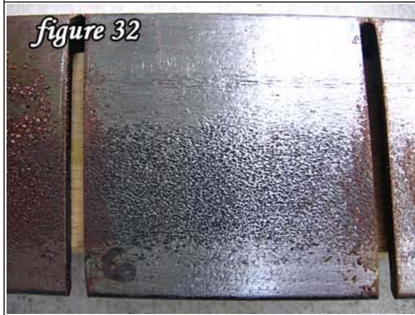
A lot of salt still remained after cleaning and formed very evident rust droplets.
