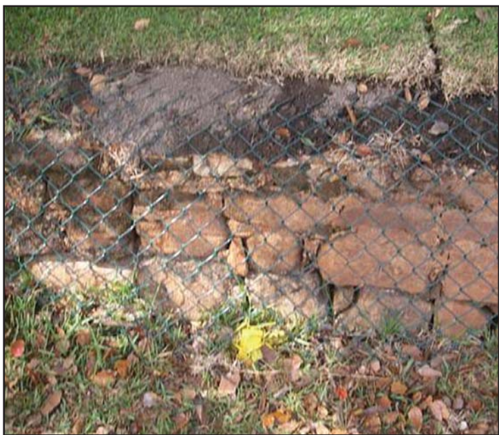
Large sections of a brick wall were unstable
