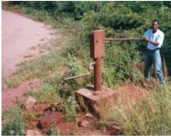
A communal pump is not as attractive as a tap at home. Photo: Rob Hope
