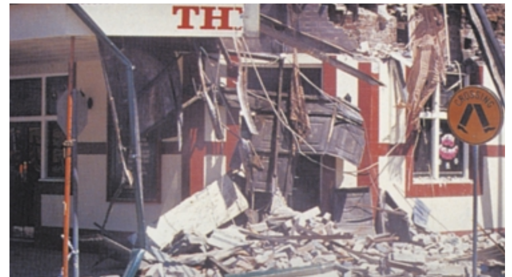
SEVERE DAMAGE TO THE KENT HOTEL, NEWCASTLE, 1989.
