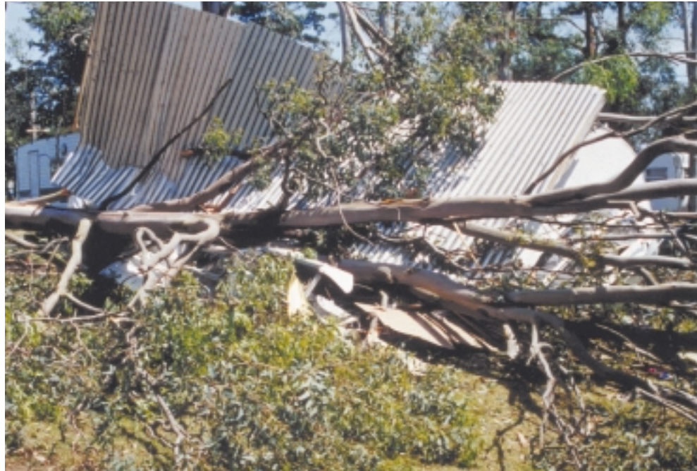
EXTREME WIND GUSTS CAN BE STRONG ENOUGH TO CAUSE SIGNIFICANT DAMAGE. AT THEIR MOST VIOLENT, THESE GUSTS ARE KNOWN AS MICRO-BURSTS AND DOWN-BURSTS, AND CAN SNAP LARGE TREES AND DEMOLISH BUILDINGS.
