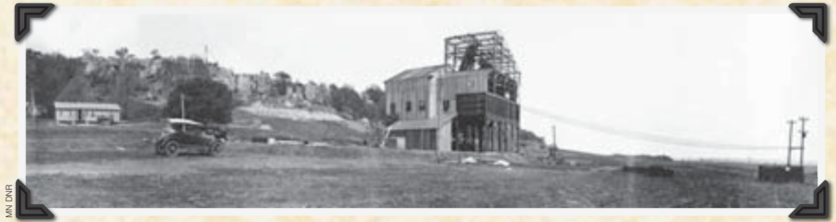
Quartzite Quarry Company crushing plant under construction in 1919. At its peak operation the Quartzite Quarry Company employed 32 men and could crush hundreds of tons of rock a day.
