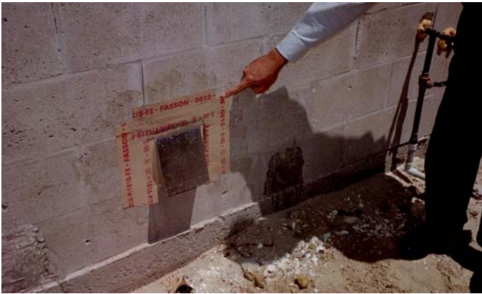
Figure 16: Membrane flashed exhaust vent
