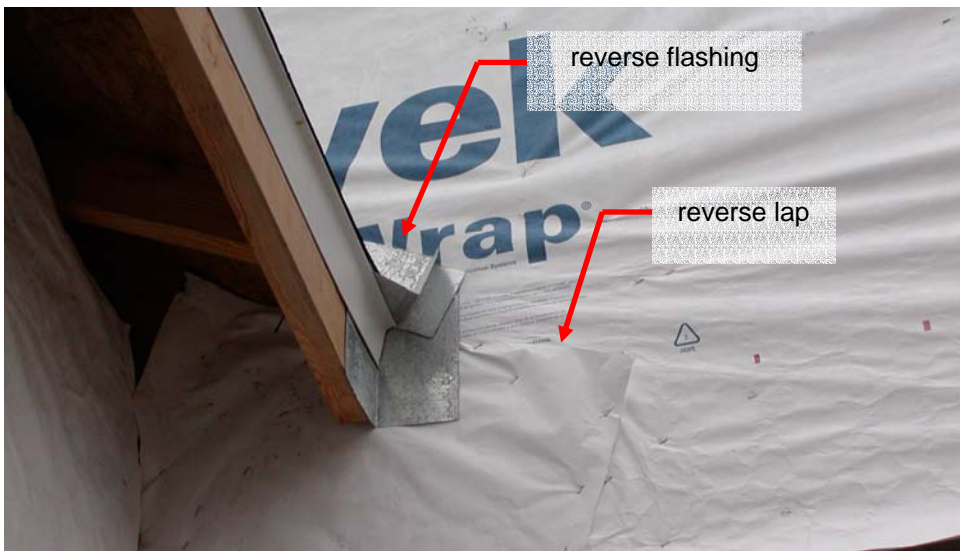
Figure 2: Improper installation of drainage plane materials
