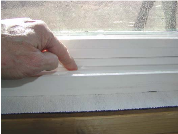
Figure 19: Water intrusion through the window frame
