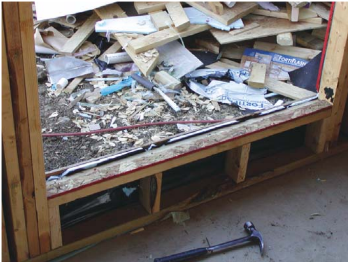
Figure 25: Drainage blocked due to exterior sheathing above the sill framing
