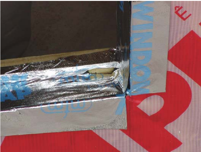
Figure 27: Torn membrane pan flashing
