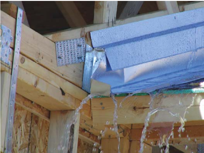
Figure 13: Poorly folded kick out flashing
