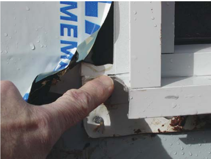
Figure 22: Cracked nailing flange at corner connection
