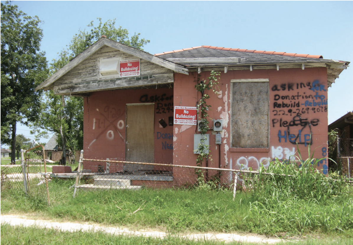
Lower Ninth Ward, August 2007. Shortfalls, delays and mismanagement of federal programs have kept money from flowing to home rebuilding and other Gulf Coast recovery efforts.
