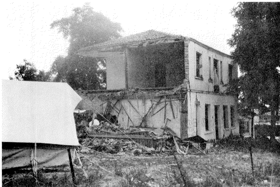
Figure 23. Fall of an exterior wall of a house at Stivos Village.
