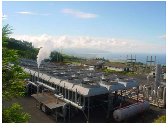
FIGURE 12.9 Two-phase binary geothermal power plant on São Miguel Island, Azores (Source: YRE International Mission in Azores—FEE Portugal).
