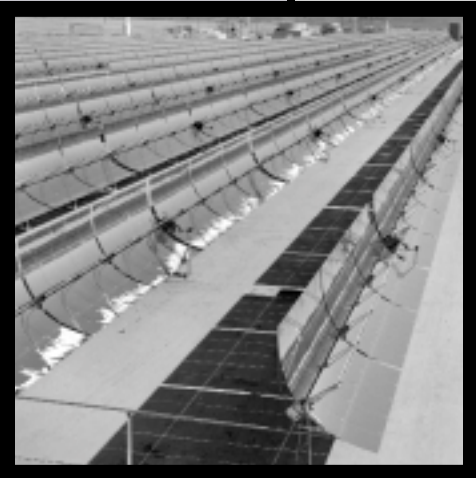
This solar power plant located in the Mojave Desert in Kramer Junction, California, is one of nine such plants built in the 1980's. During operation, oil in the receiver tubes collects the concentrated solar energy as heat and is pumped to a power block located at the power plant for generating electricity.
