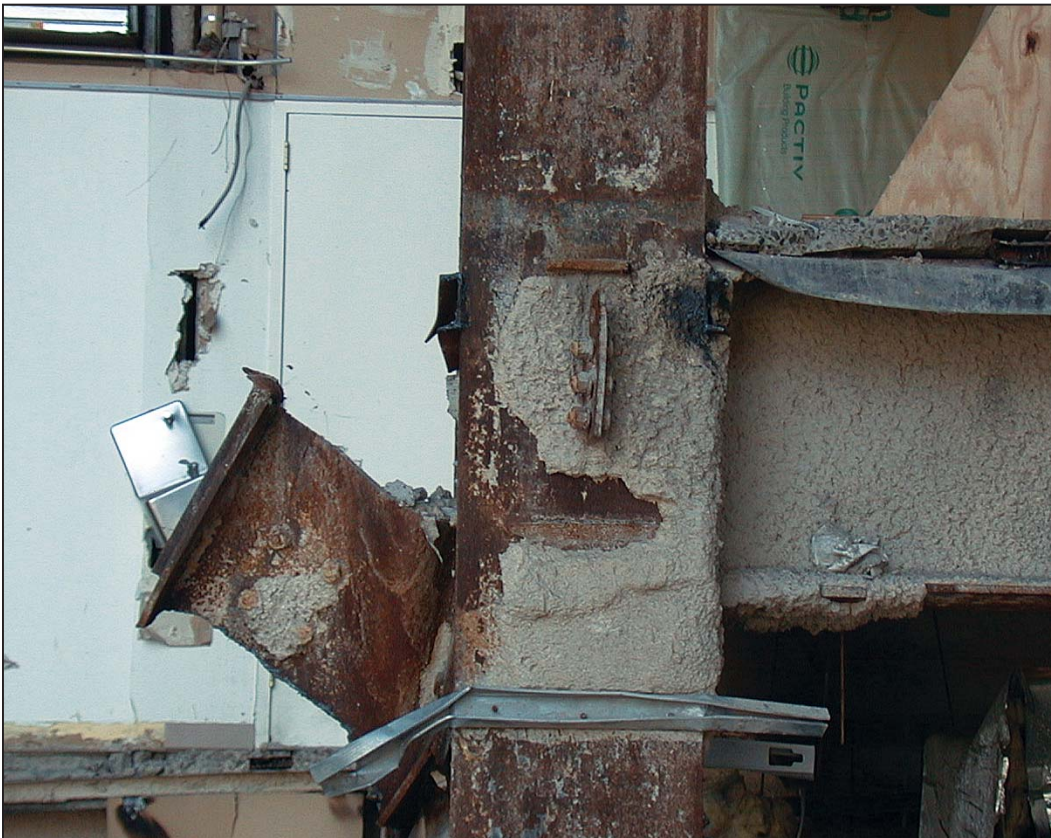
Figure 6-7 Column with the remains of two moment connections.
