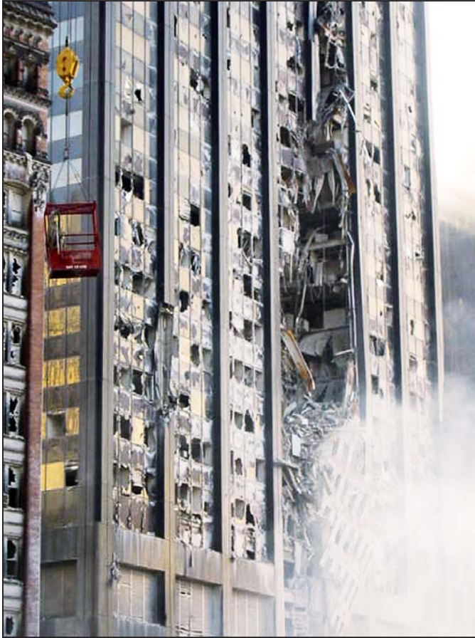
Figure 6-2 Closeup of area of partial collapse. Note debris accumulated at the bottom of the damage area, resting on the 8th floor. Area of initial impact is not shown in this photo.
