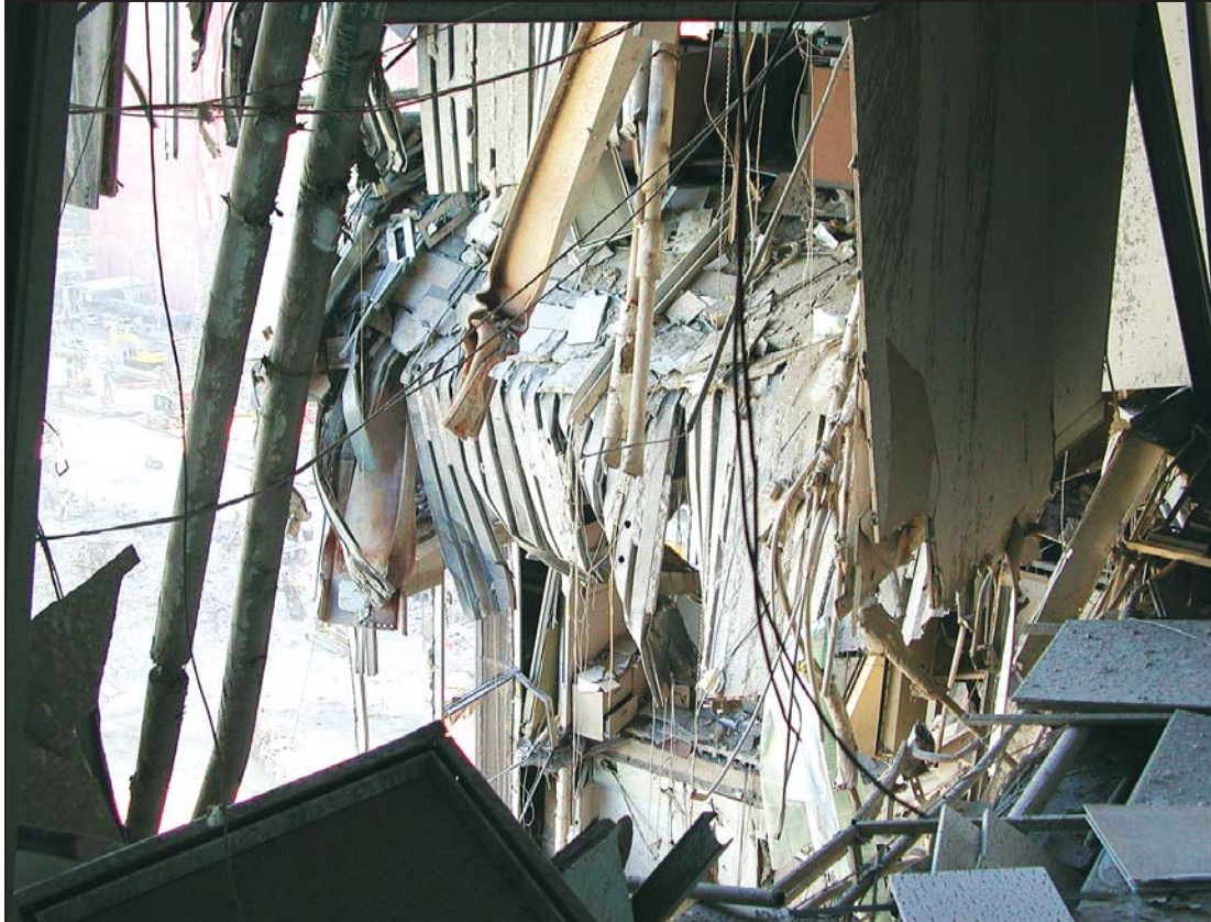
Figure 6-10 Area of collapsed floor slab in bays between C-8, E-8, C-7, and E-7, from the 15th floor.
