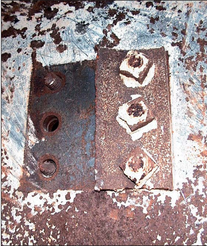
Figure 6-8 Failed shear connection of beam web to column web.
