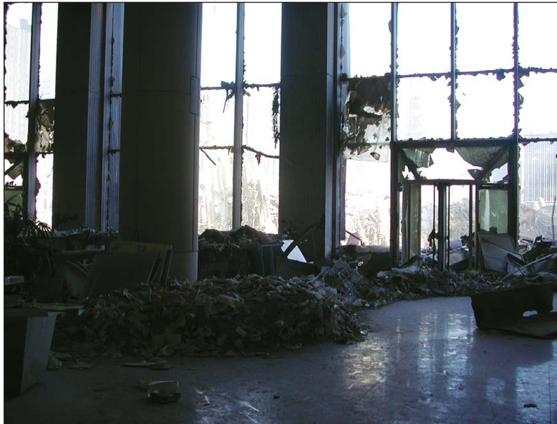
Figure 6-11 Bankers Trust lobby (note debris has been swept into piles).
