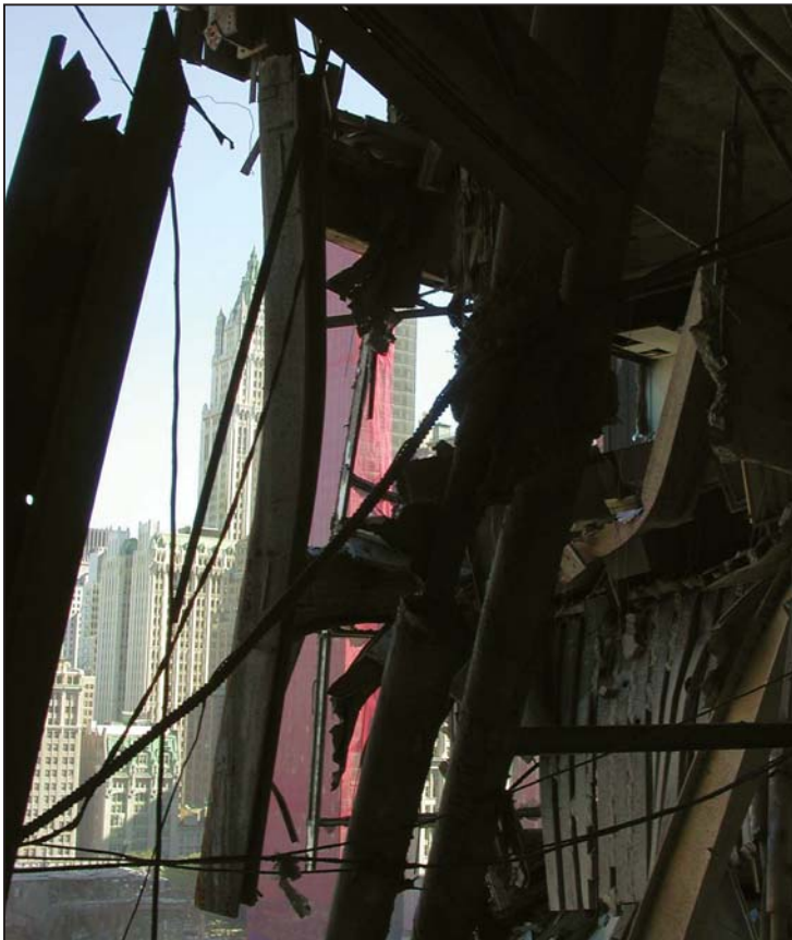
Figure 6-9 Suspended column D-8 at the 15th floor. Note separation at column splices.
