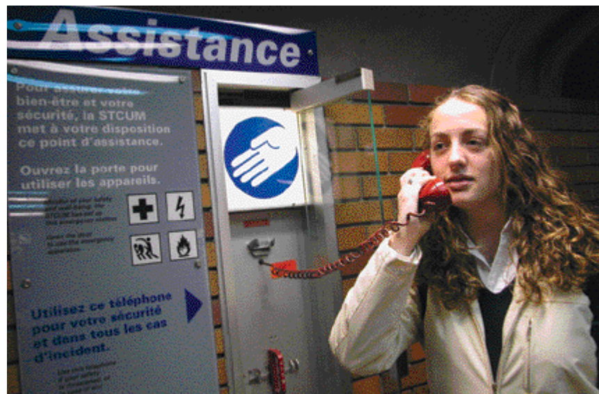
Each train platform holds at least one emergency telephone linked directly to the Control Centre. (Michel E. Tremblay - STM)
