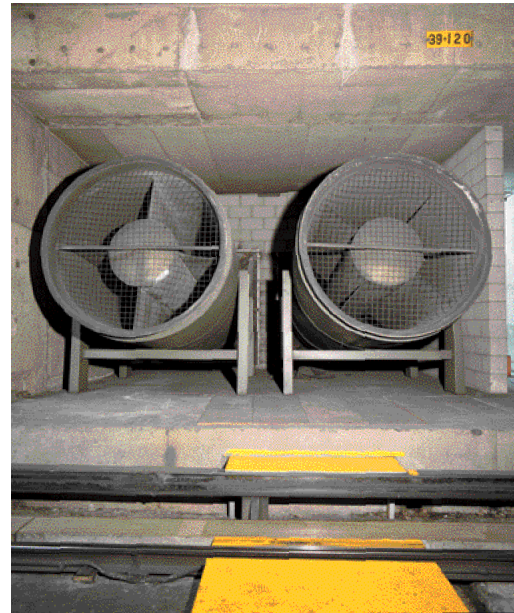
Ventilation units inside tunnel. (STM Archives)
