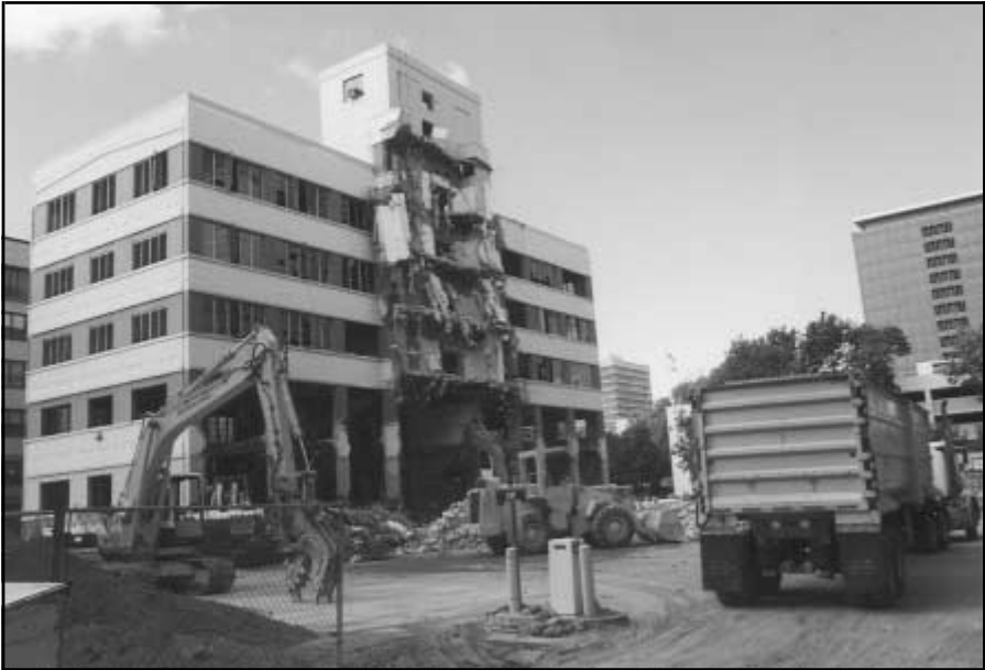
A portion of the LOB demolished during November 1999 remodeling Legislative Office Building (LOB)
