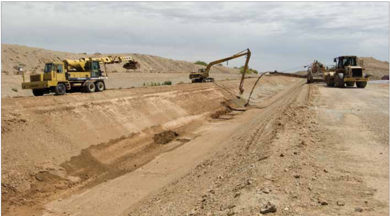
R&L Brosamer, Inc., is building a new, 35-mile section of concrete lined waterway parallel to the existing Coachella Canal. When complete, the new section will replace the last remaining unlined section of the 122-mile canal.
