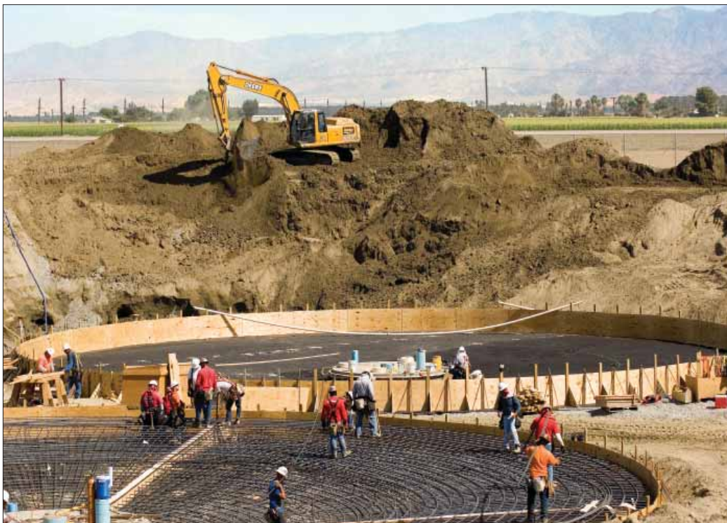
The wastewater reclamation plant in Thermal is being expanded to keep up with growth in the surrounding area. The plant soon will be able to accept 7 million gallons of wastewater daily.
