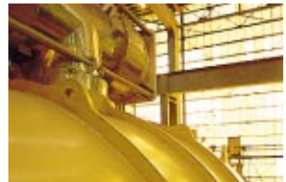
Tarong Power Station's turbine hall.
