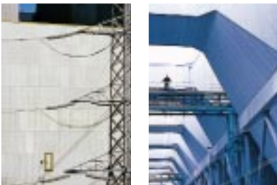
Transmission lines linking to the electricity grid at Tarong (left) and electrostatic precipitators.
