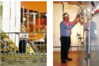
Key Radloff inspecting the generator circuit breakers at Wivenhoe (left), while Ray Morton tests the battery charger operations.
