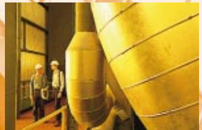
Allan Kirsch (left) and Glen Lumsden inspecting a feed water tank in the turbine hall.
