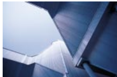
Tarong Power Station's electrostatic precipitators.
