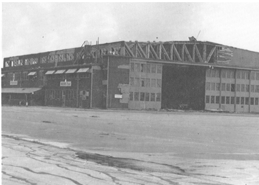
Hurricane damage, Homestead Army Airfield, September 1945
