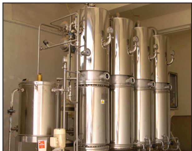
High grade water production plant.
