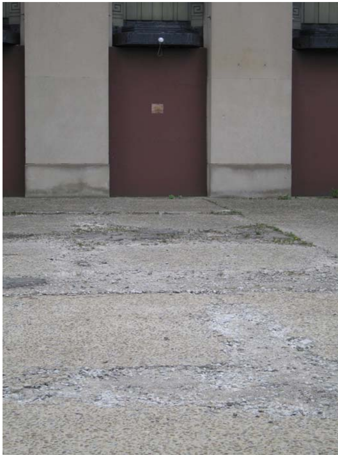
Crumbling sidewalk at the entrance to the Aud
