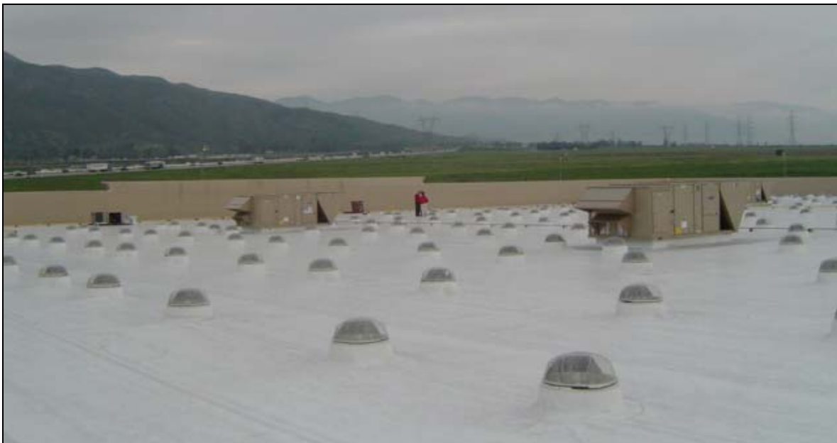
Solar tubes direct sunlight energy into the Fontana North (California) Target store.
