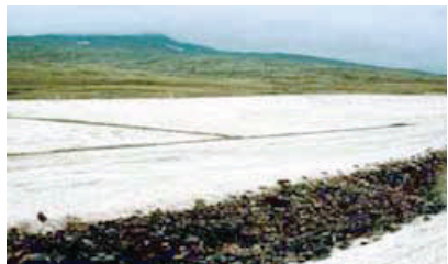
Figure 89: Well-placed excelsior blankets being used to control erosion prior to vegetation growth.
