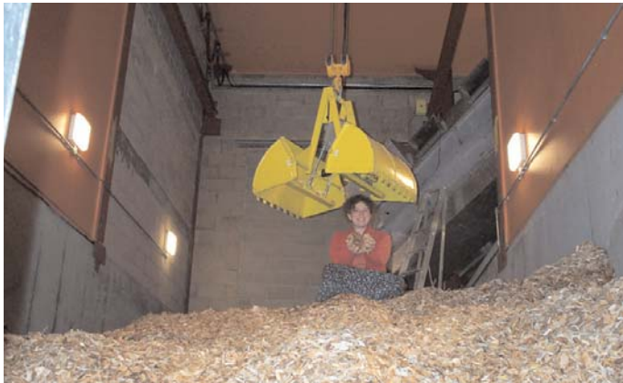
BedZED's wood chip combined heat and power unit
