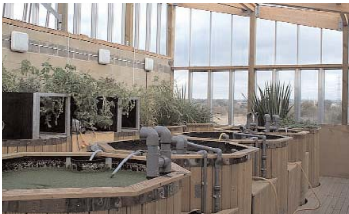
BedZED's living machine on-site sewage treatment plant
