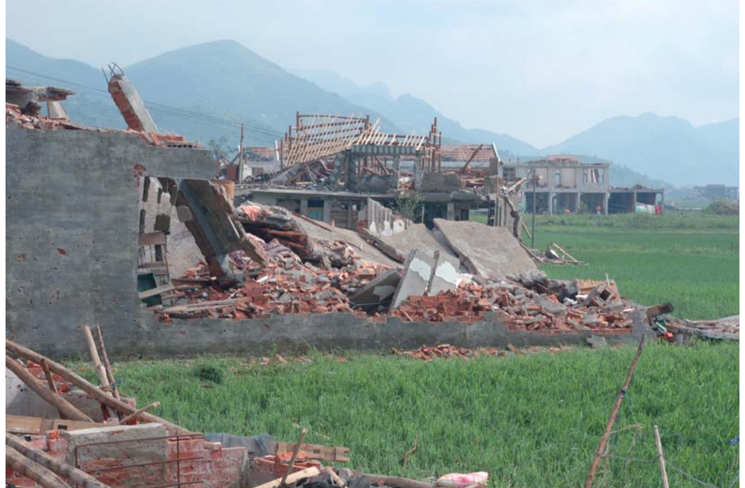
FIGURE 29: BUILDING DAMAGE IN ZHEJIANG PROVINCE
