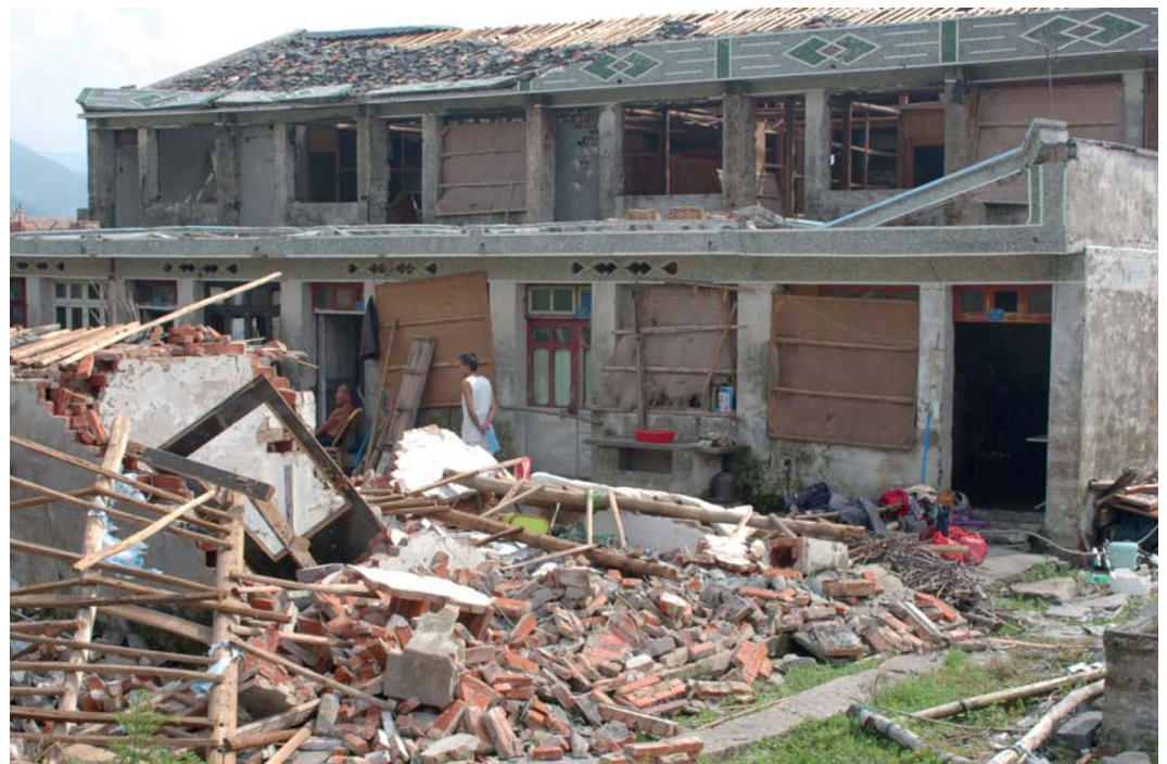
FIGURE 27: TYPHOON SAOMAI RIPPED ROOFS OFF PROPERTIES AND BLEW IN WINDOWS, CAUSING EXTENSIVE STRUCTURAL DAMAGE IN SOME PLACES
