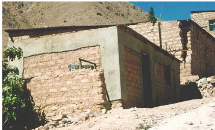
Figure 22 – A House with External Welded Mesh Reinforcement Remained undamaged (front) whereas a House Without Reinforcement (shown at the back) was Severely Affected by the 2001 Arequipa Earthquake, Peru (Zegarra et al, 2001)
