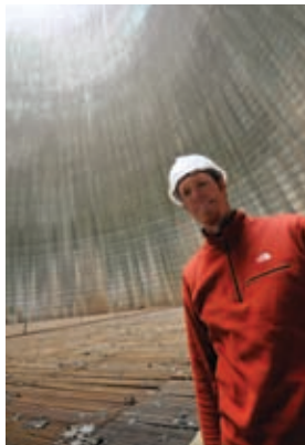
Above: Sean Riley checks out the inside of a cooling tower at Susquehanna Nuclear Power Plant.
