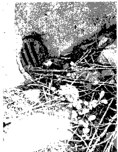
Figure 32 Drainage of the emplacements has been reduced by blocked drains (bay B), Salmond Reed 1003
