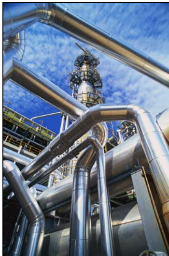
Wastewater Treatment Plant.
