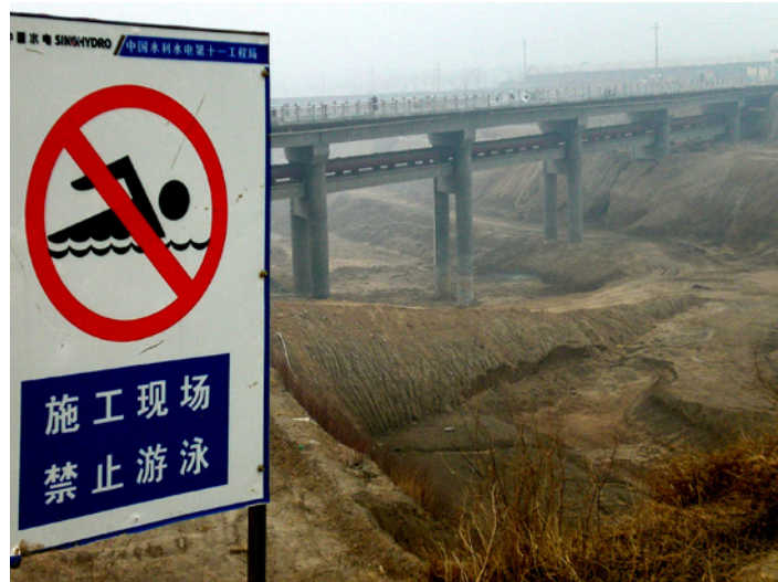
One of the massive canals being constructed for the South–North Water Diversion project in China.
