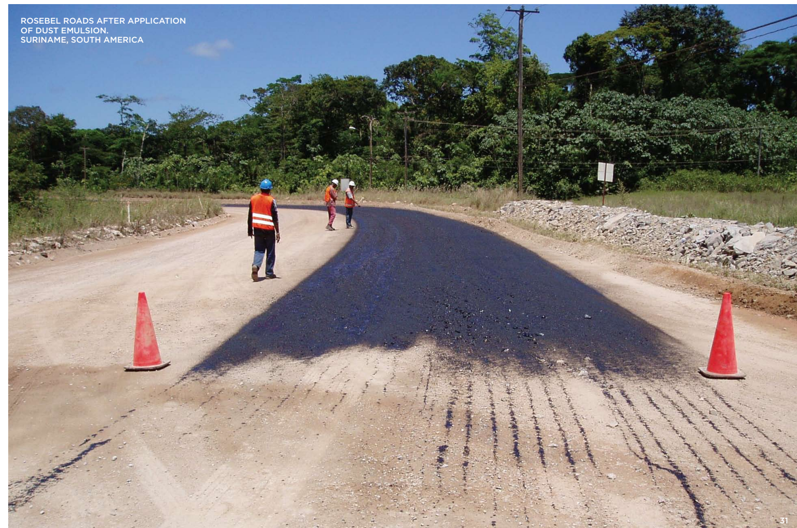
DUST STABILIZER EMULSION (DSE) IS APPLIED ON ROADS AT ROSEBEL GOLD MINE. SURINAME, SOUTH AMERICA
