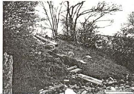
Above: Shoreline along Lake Poinsett before stabilization.
