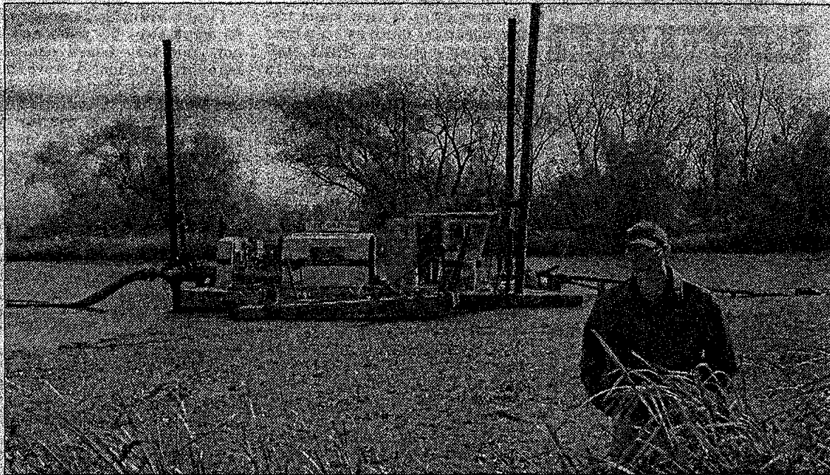
Jason Venjohn stands in front of the dredge barge on Oct. 15 as the work crew rushes to get as much done as possible before the cutoff day on Sunday, Oct. 17. (More photos on page 3)
