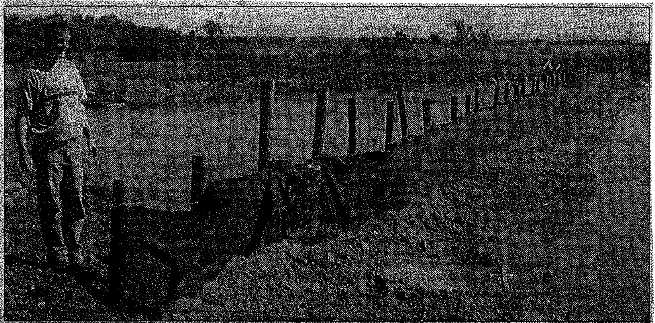
Clean water returns to the lake through this filtration screen. The clean water return culvert is just to the right of Lake Project Coordinator Kevin Stark.
