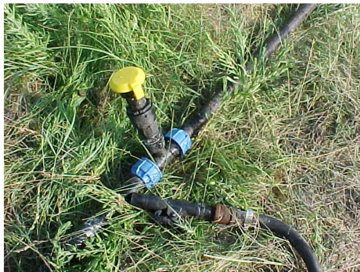
Figure 3. Above ground pipe and quick coupler.
