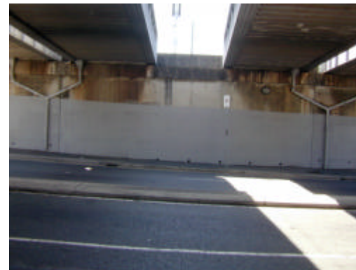
Photo 22 - the standard colour should be applied to a minimum of three (3) metres from the ground.
