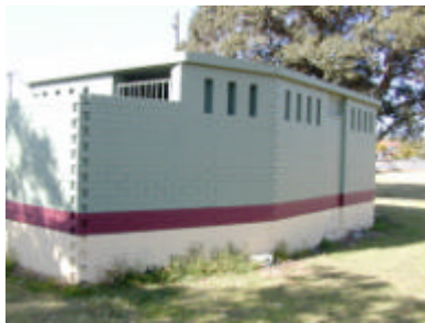
Photo 20- graffiti masking is very difficult when a structure has a blend of colours. In this case a reliable protective coating would be required.
