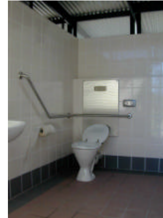
Photo 23 - tiles are hard and are quite easy to clean graffiti from. The major problem is that paint easily soaks into the grout.
