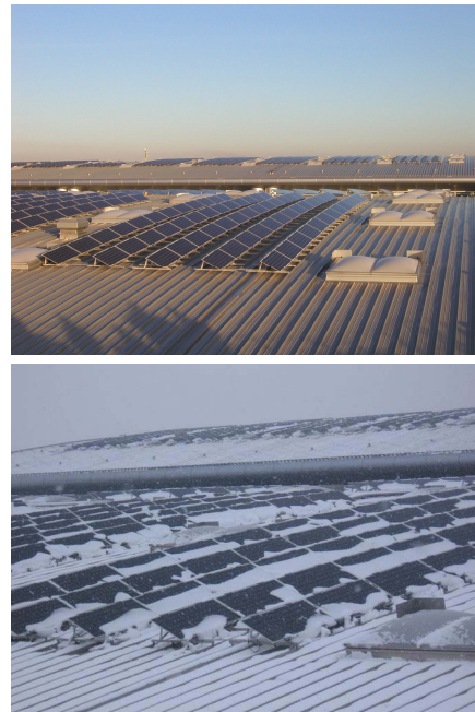
Figure 2 and 3: Modules of the 1 MW p system in summer and winter
