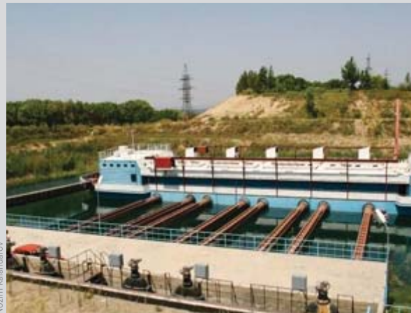
This pump station supplies precious water for rural poor
