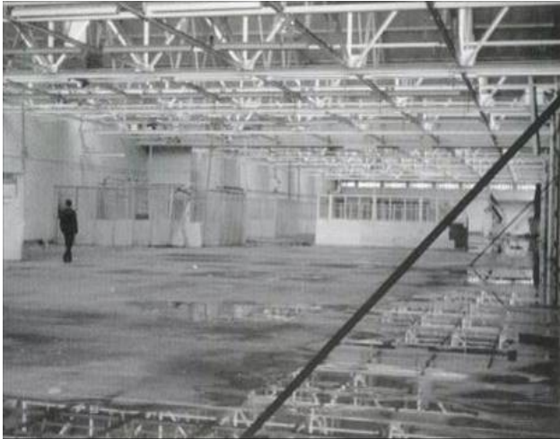
Before the hole in the roof was fixed.....
