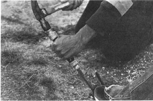
Place the driver over the sharpened end of the rebar stake and hammer it in.
