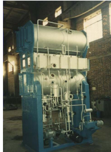
70kW two stage absorption chiller ( Guangzhou, China, 1994 )
