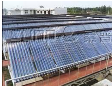
Solar cooling Project in Qingdao
