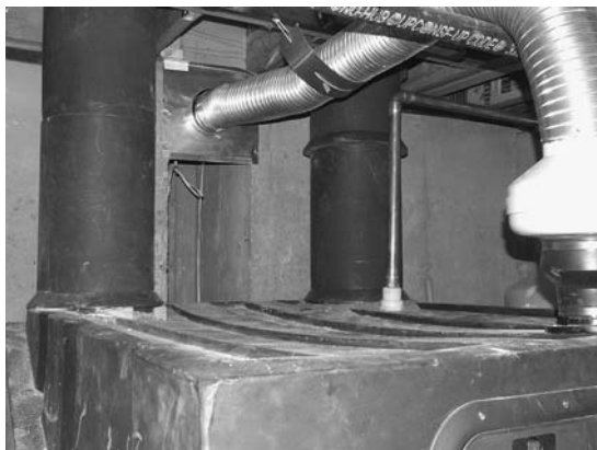
FIGURE 8. Compost Toilet—Chutes, Exhaust.
