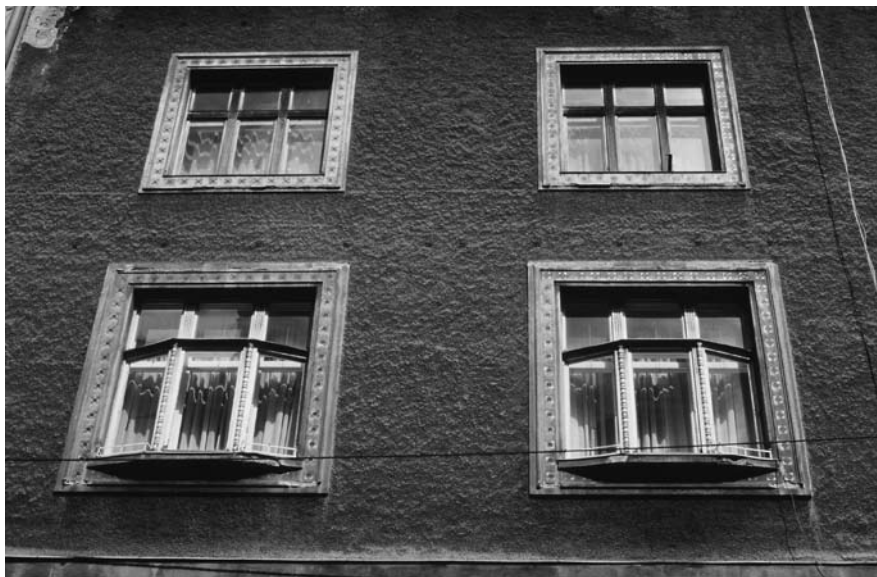
Trgovačko-stambena kuća Pavelić, Masarykova 8, Zagreb (foto: M. Drmić) Commercial and residence building Pavelić, 8 Masarykova Street, Zagreb
