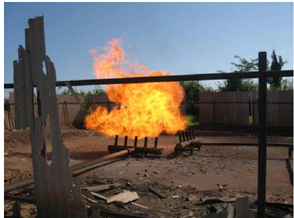
Ground flare without proper enclosure at oil mining site at Arunachal Pradesh
