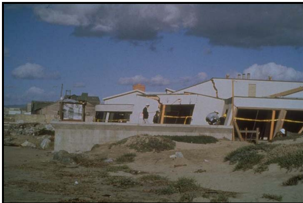
1989 Loma Prieta Earthquake – Moss Landing Marine Laboratories Showing structure “stretched” more than 5 feet due to lateral spreading
