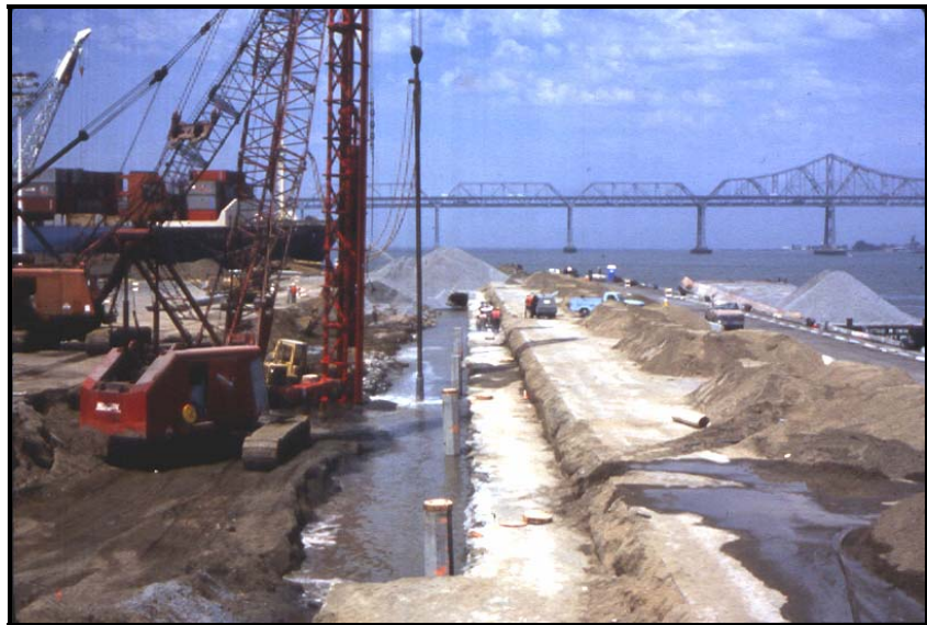
Pile installation work at Port of Oakland 7 th Street Marine Terminal Source – J. Egan, Geomatrix
