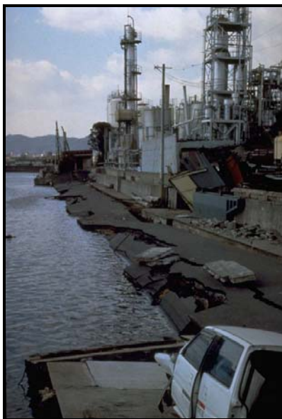
1995 Kobe Earthquake – Example of damage to port facilities
