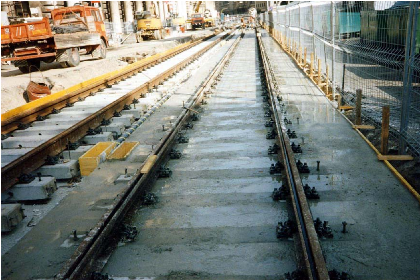
FIGURE 6 Piazza Vittorio Emanuele under construction. On the left, the first layer of concrete has been laid. On the right, the second layer of concrete has been laid, up to the top level of the concrete sleepers.
