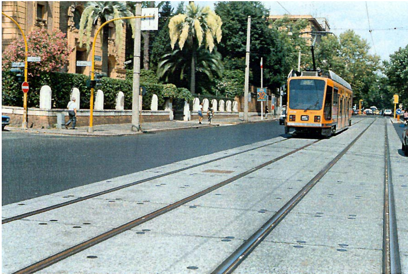
FIGURE 4 The final result of the works with vehicles operating revenue service on Viale Regina Margherita.
