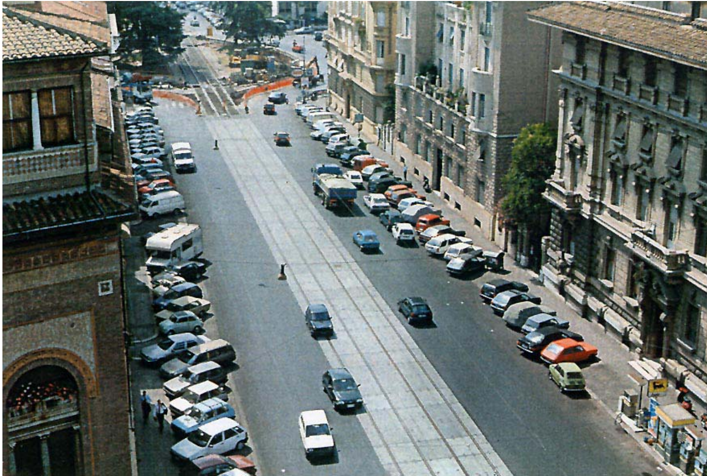
FIGURE 3 Aerial view of the construction site (last phase) on Viale Regina Margherita.
