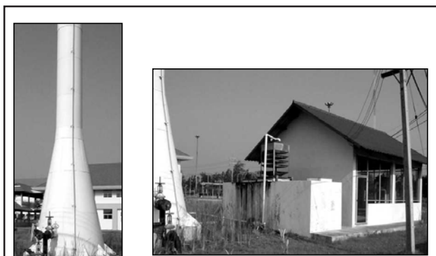
Figures 2a and b. Rajasuda College water tower and pump house with aerating system. Buddhamonton, Nakhon Pratom, Thailand.
